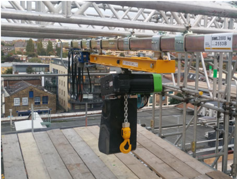
Typical Hoist and Winch project - a 2000 kg Swl Single fall hoist incorporated onto a special scaffold structure and used in the refurbishment of a five storey building in central London.
