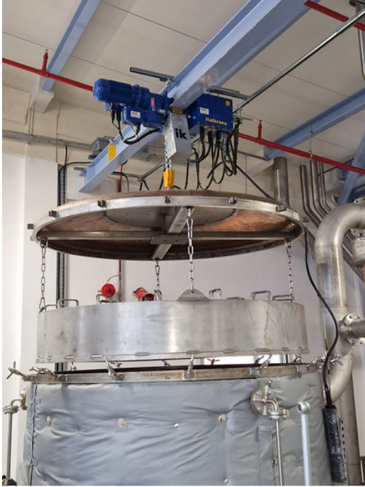
The 2-ton swl (safe working load) hoists raise and lower sealed vessel lids and baskets containing raw materials used in the production of gin.
