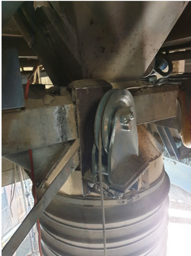
Export chute winch - typical pulley mounting.
