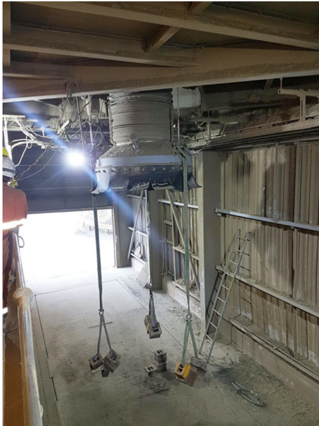
The telescopic export chute in raised position under proof load test.
