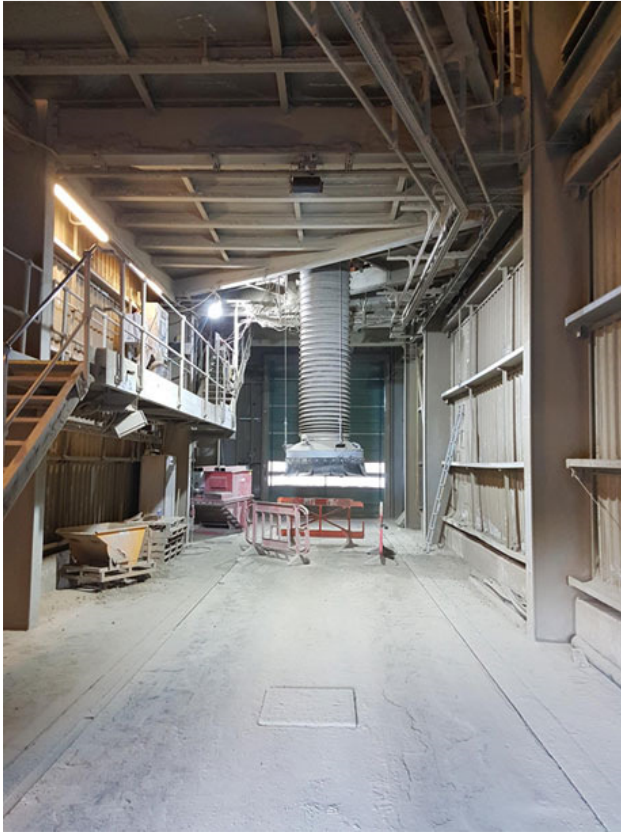
The telescopic export chute in lowered position.
