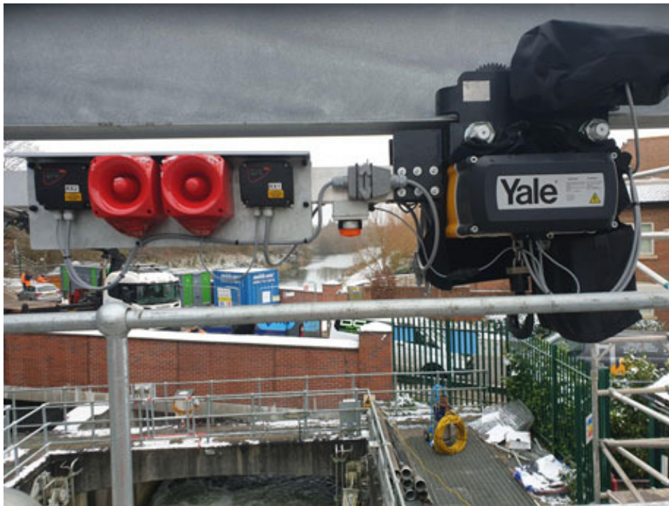
Tandem hoist control board with radio receivers.
