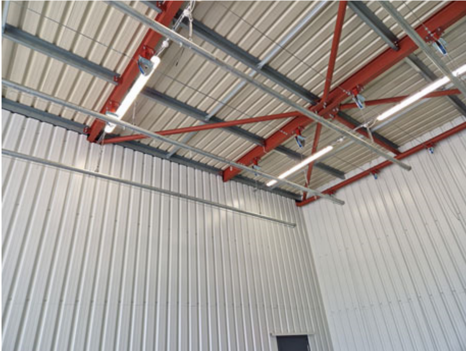
Diverter pulley and spreader beam installation on a bespoke electric-powered winch lifting system undertaken by Hoist & Winch Ltd.
